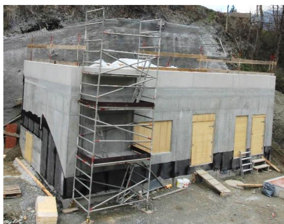
Local de turbinage – Station aval
